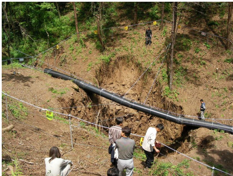
Figure 4.8. Sinkhole crater in Korea (photo by Song).
