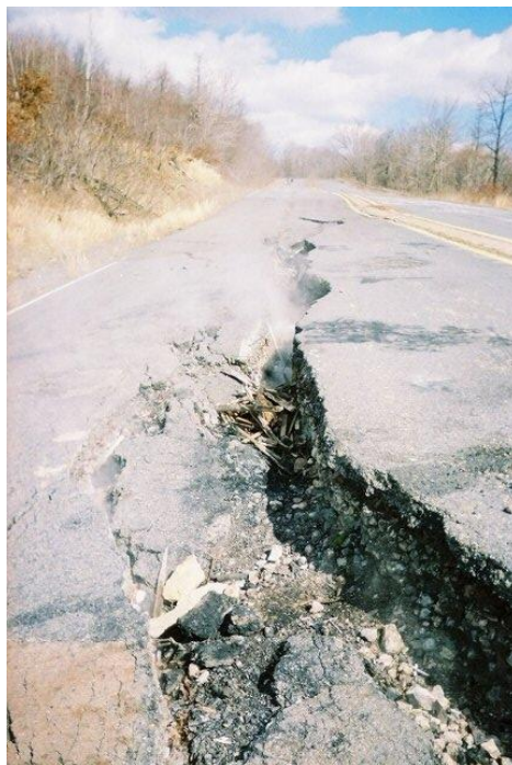
Figure 4.4. Subsidence above underground fire in Pennsylvania (USA) (Source http://www.offroaders.com/album/centralia/Jonathan_Gatarz/FL00026.jpg ).
