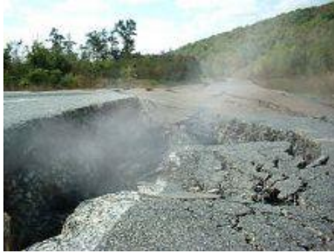
Figure 4.22. Sinkhole above underground fire in Pennsylvania (USA) (Source http://www.offroaders.com/album/centralia/Jonathan_Gatarz/FL00026.jpg )
