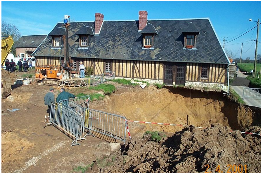
Figure 4.9. Sinkhole within urban area (Neuville-sur-Authou –Normandie – France, source CETE/MEEDAT).
