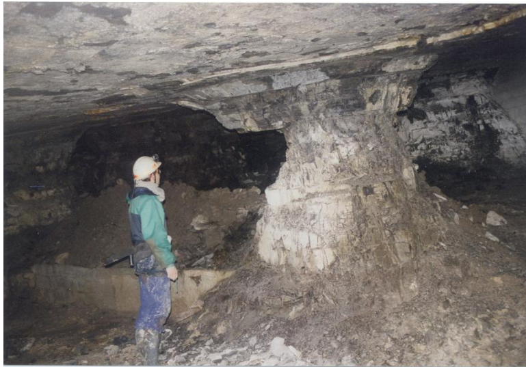
Figure 4.15. View of a degraded pillar in Provence – France (Source INERIS).
